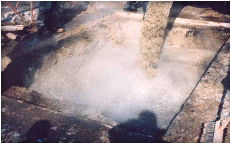
Figure 8. Low density concrete fill (unshrinkable fill) poured into a utility trench from a ready-mix concrete truck.
