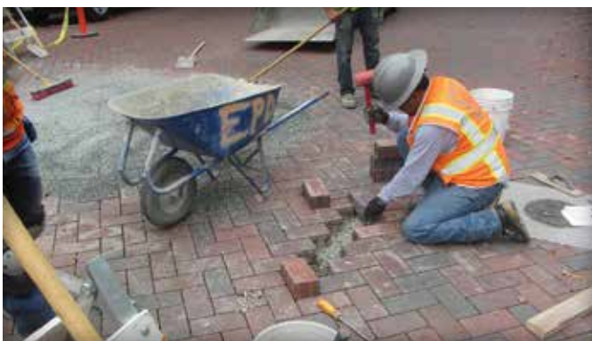
Figure 4. Reinstatement using the same pavers continues following the existing herringbone paving pattern.
