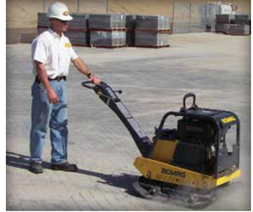
Figure 14. Second and final compaction of the pavers. The first compaction occurs after the pavers are placed (no sand in the joints). The second compaction works the sand on pavers into the joints. This process causes the pavers to interlock.
